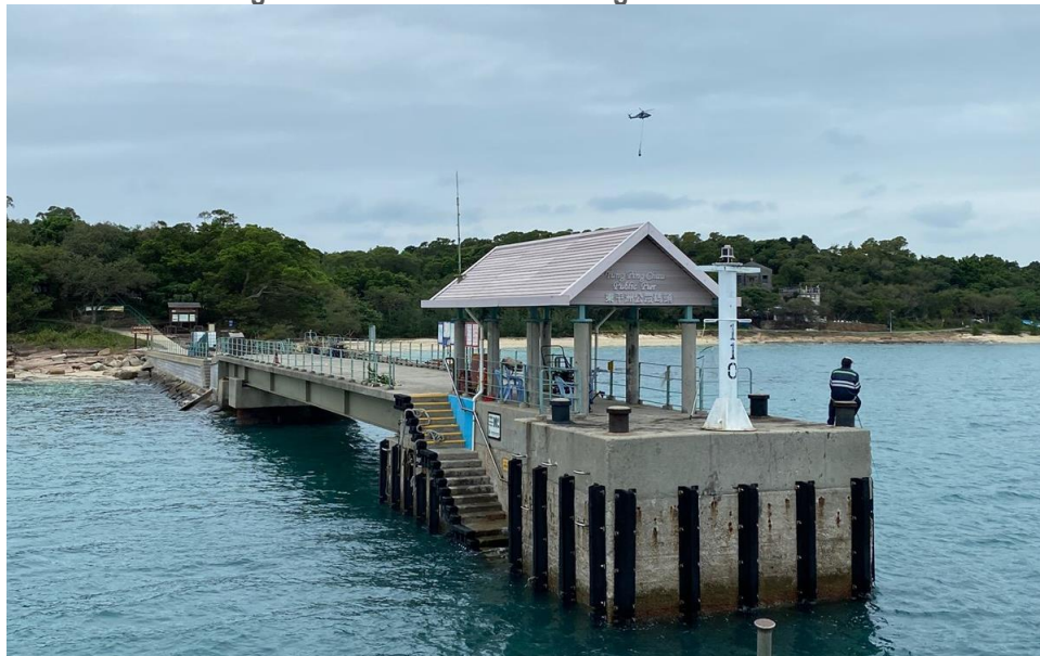
Figure 2.2: Condition of Existing TPC Public Pier
